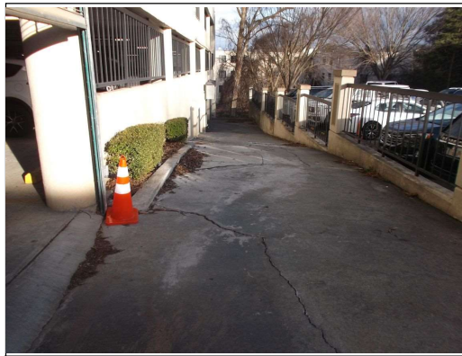
Driveway major cracks and defective repairs
