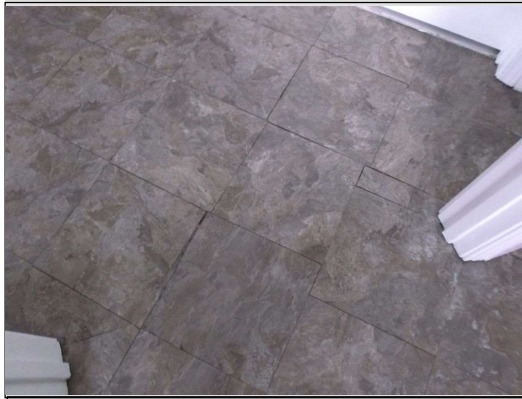
Floor tiles shifting at areas
