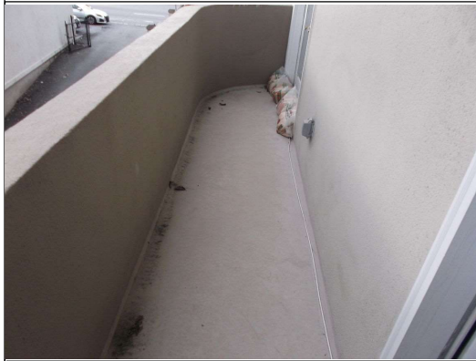
Drainage holes too small at side balcony
