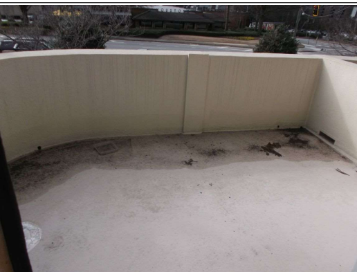
Drainage holes too small for heavy rain, debris
