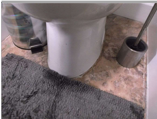
Defective caulk where the toilet rest on floor
