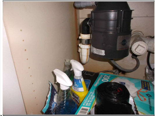
Stains on drain pipe to disposal
