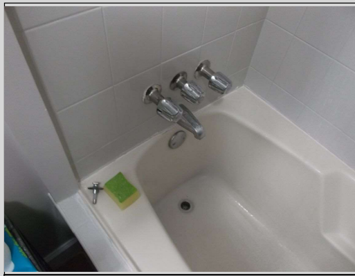
Stopper not in place/knobs loose
