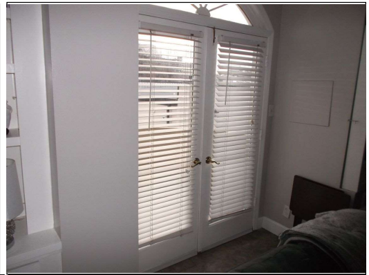
Front patio door damaged at the bottom lock
