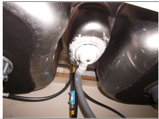
Improper drain assembly at center sink
