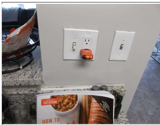
Receptacle did not trip when tested
