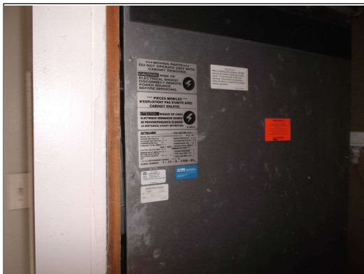
Furnace electric in closet
