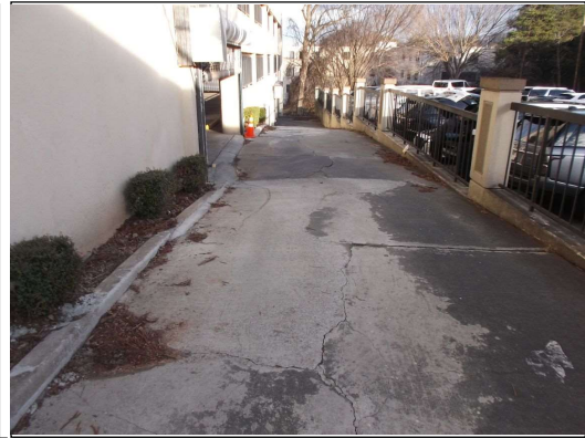
Driveway cracking and defective patches
