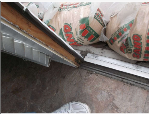
Front fixed door slab split at the lock
