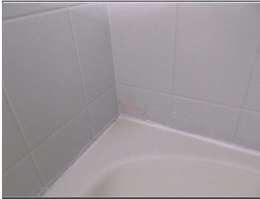
Defective glaze on tiles
