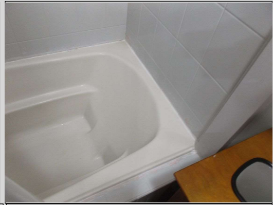
Defective caulk at tile and tub
