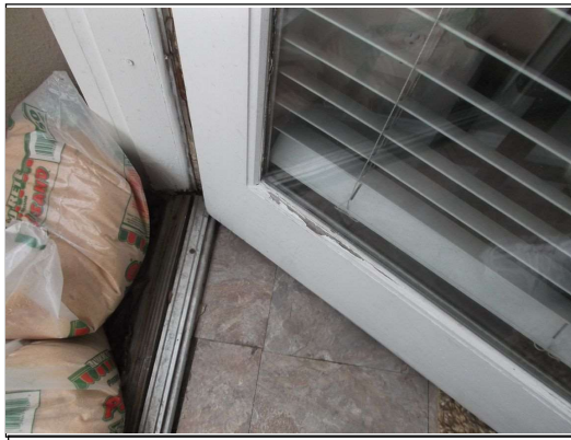
Exterior doors may need paint in near future
